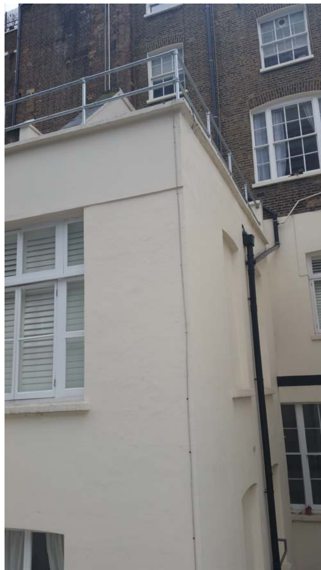
VIEW FROM FIRST FLOOR LEVEL OF 101 EASTBOURNE MEWS LOOKING OUT TO 101 WESTBOURNE TERRACE.
